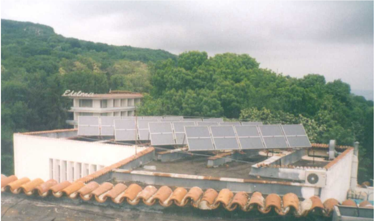
Solar collectors in Horizont Hotel – Golden Sands Resort, mounted by “Anita” Company
