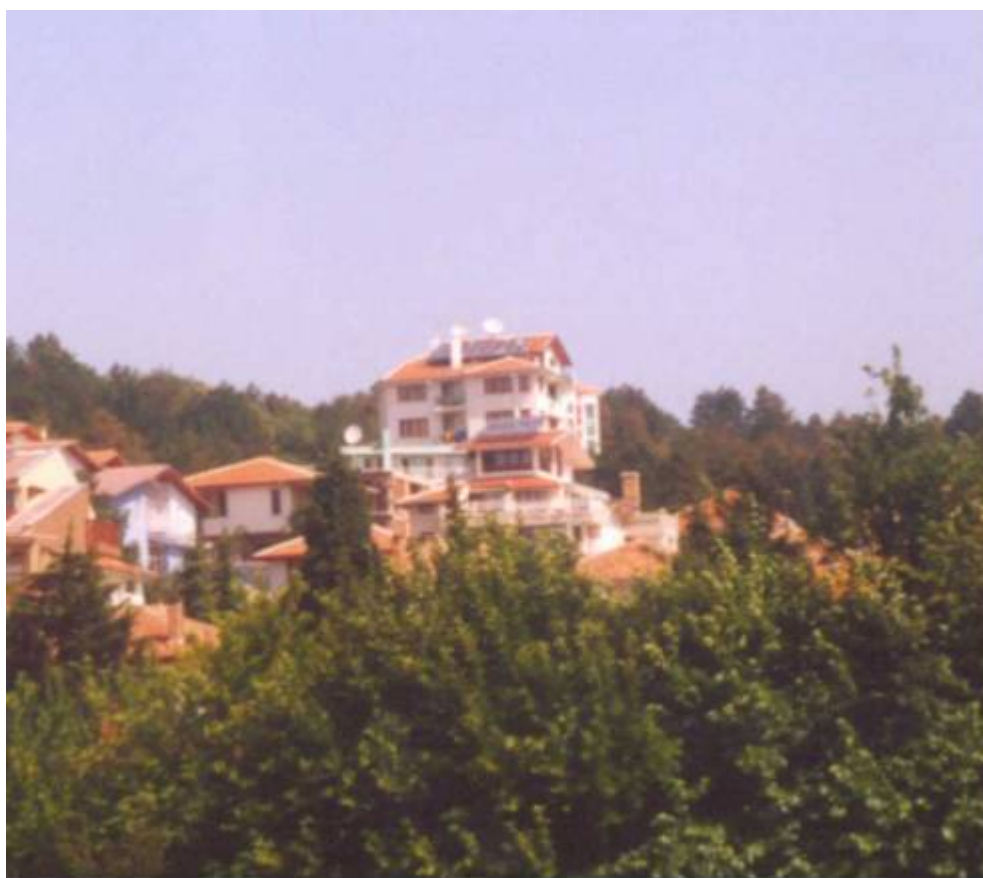
Photo 3.1 Hotel “Zora” in Sunny Beach, equipped with a solar system (27m 2 /2000l)
